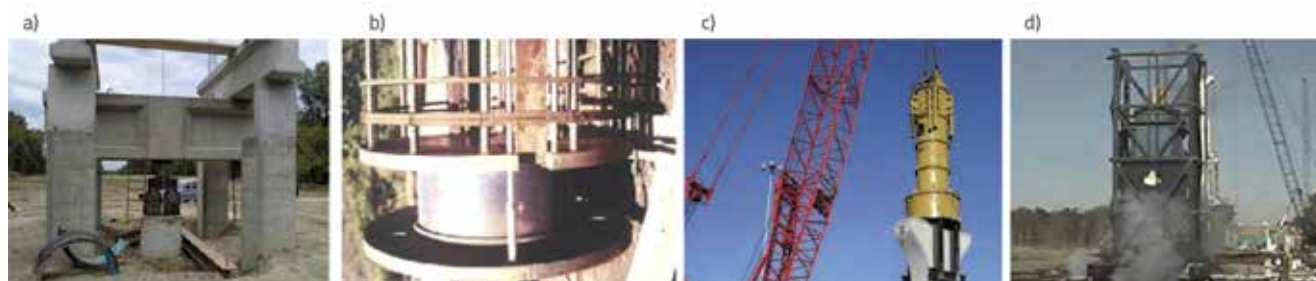
Figure 9. Field testing of pile capacity by: a) static testing; b) Osterberg cells; c) dynamic testing; d) Statnamic testing [9]
