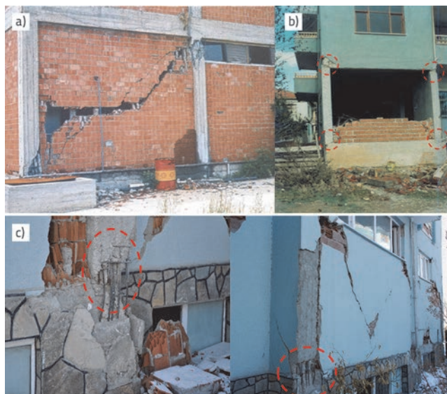
Figure 1. Damaged infilled frame: a) 1998 Adana-Ceyhan earthquake [3]; b) 1995 Dinar earthquake [4], c) 2011 Van earthquake
